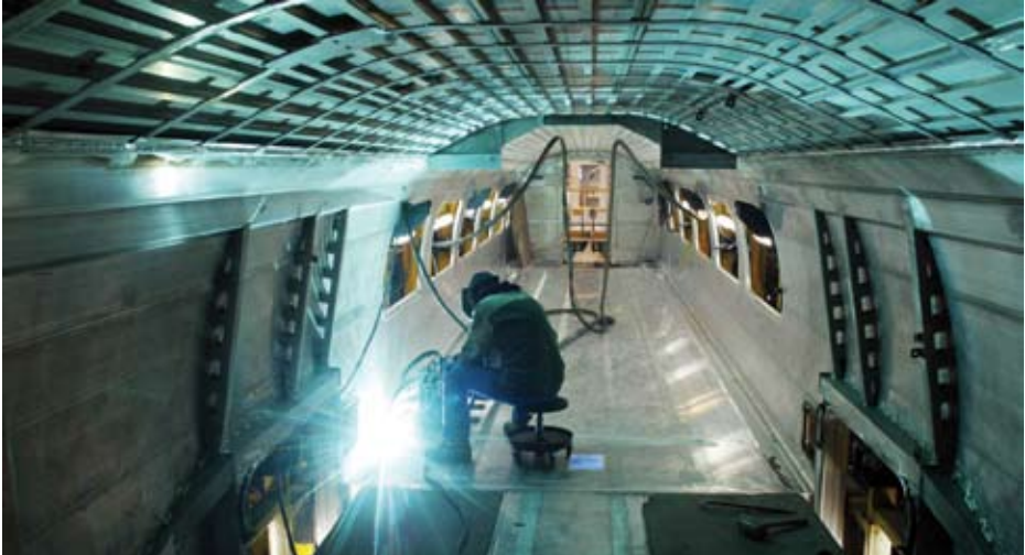
An Alstom hydropower equipment plant in Malaysia steps up the pace
